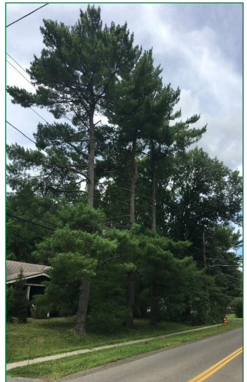
Photograph 4. Trees along ROW where powerlines are conflicting.
