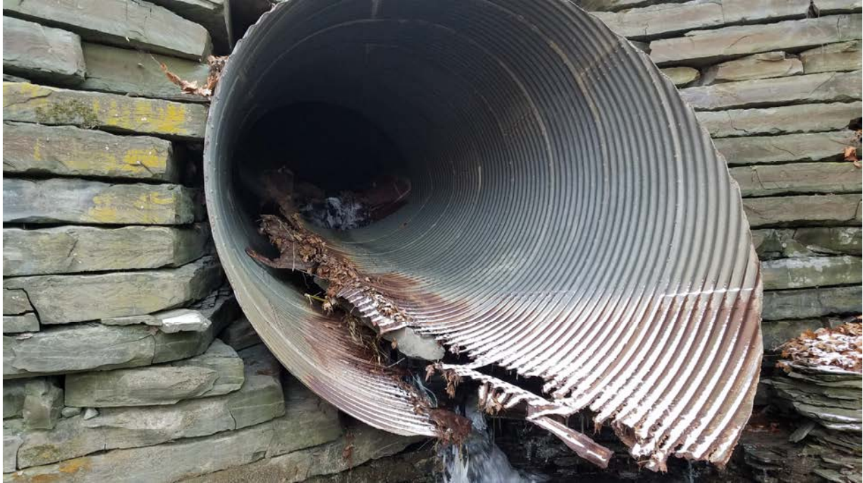
Photo #3 – Outlet End of Pipe – Rotted pipe folding in on itself
