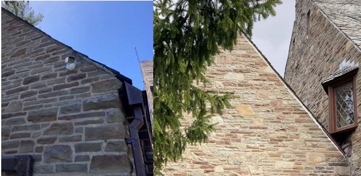
Mortar joint separation between the wall and roof on the northeast wall of Section F (L) and the southwest wall of Section B (R).
