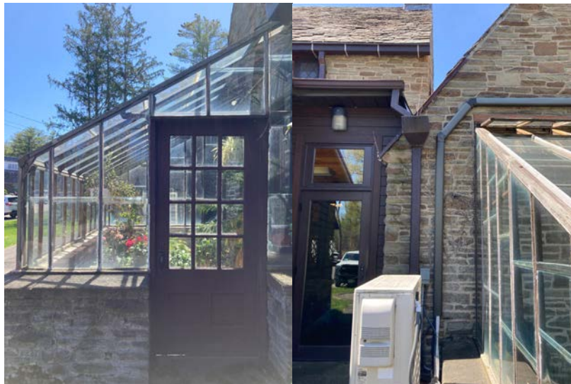
Section D, facing northwest (L), and abutting E (R). For a full view of the greenhouse, see Section B.
