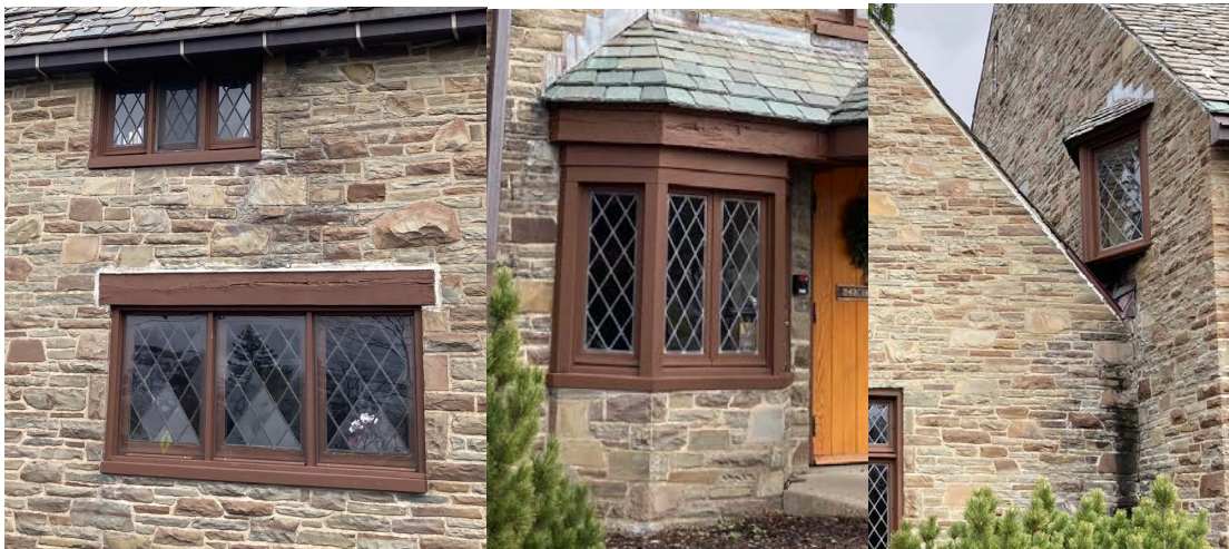
Moisture damage and staining between the eastern windows on Section A (L), next to the western oriel (C), and at the junction of Section A and B (R).
