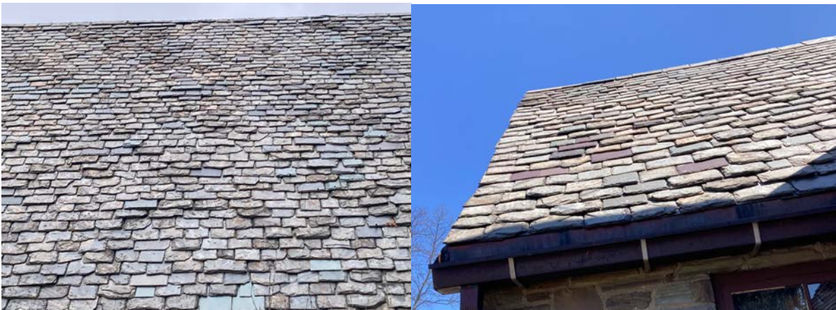
Slate shingle condition along the southeast elevation of Section F (L) and the southwest elevation of Section C (R), showing delamination and the piecemeal addition of new shingles.
