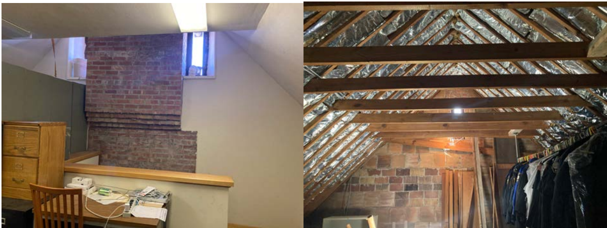
The finished (L) and unfinished (R) gable ends of the attic, with the exposed chimney in the finished section.
