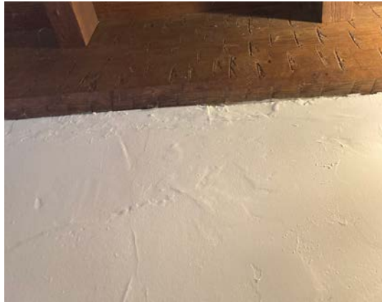
Bubbling and chipping of the plaster where it meets the wood member in the lobby.
