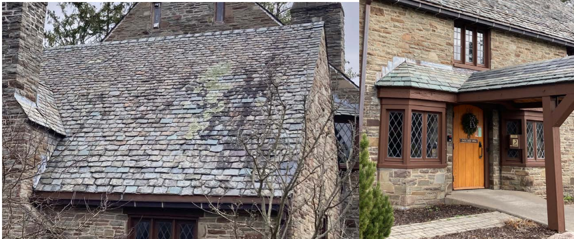
Black and green biological growth on the northwest roof of Section B (L). Rust stains on the shingles of the portico (R).
