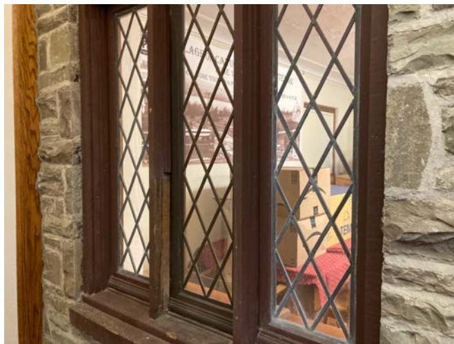
Chipping and wear on the original exterior windows outside the Jury Room.
