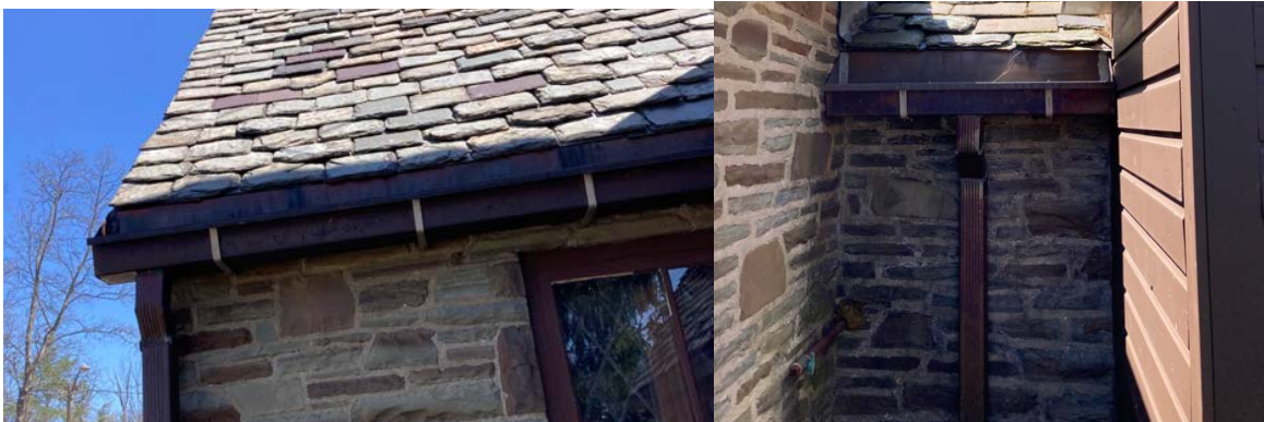
Rusted gutters around Section C and the hyphen.
