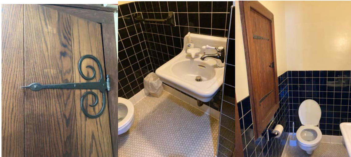
Village Court bathroom, door detail (L), sink (C), and toilet and medicine cabinet (R).
