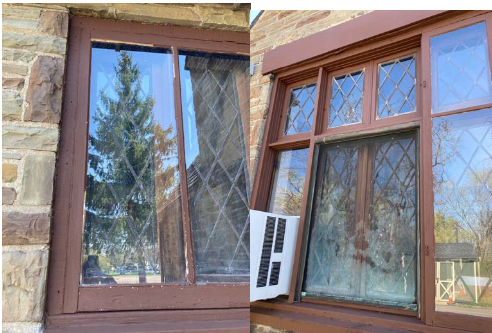
Broken storm window and paint chipping on the southwest elevation of Section C, and deterioration of the window on the northwest elevation.
