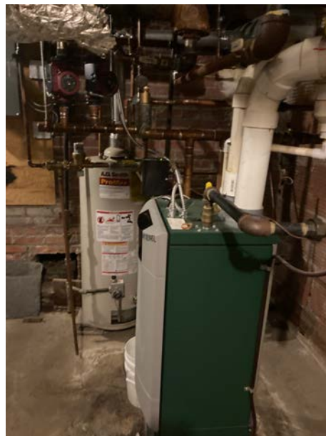
Basement, natural gas hot water heater and reservoir.
