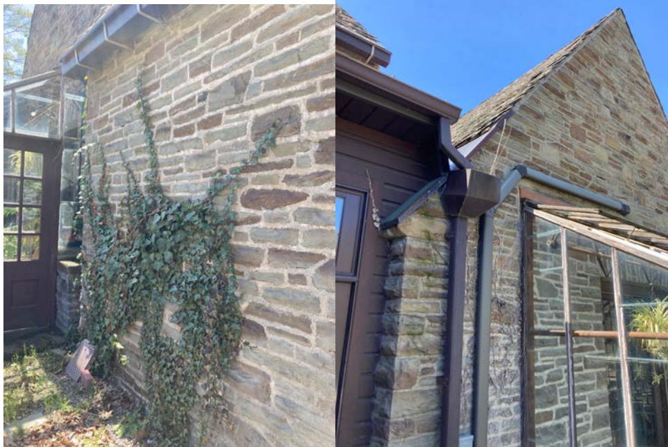
Vegetation growing along the northeast walls of Section C (L) and Section B (R).
