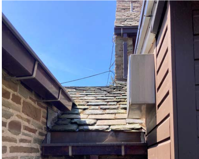
Accumulated biological detritus and yellow-green biological growth on the northeast roof of the hyphen.
