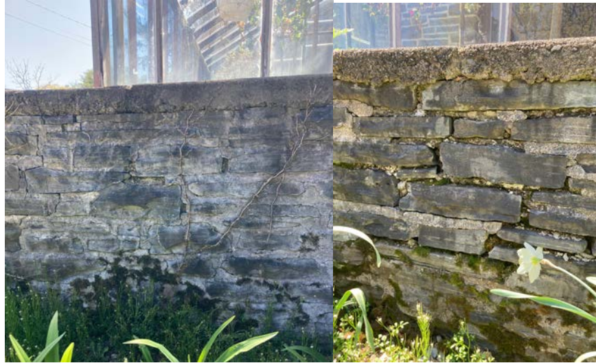
Poor condition of the stone half-walls of Section D.
