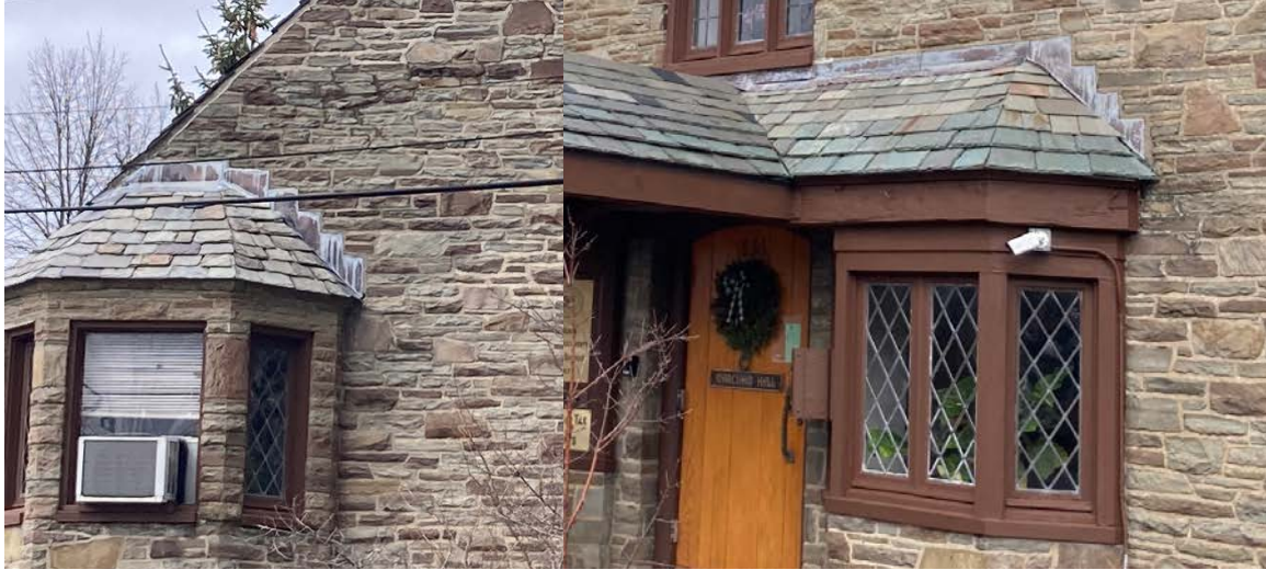
Rust on the flashing above the bay projection (L) and the portico (R).
