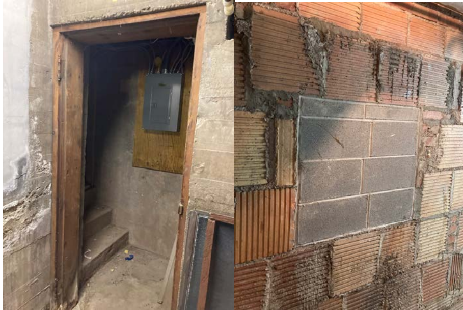
Deteriorated concrete in the basement (L) and clay tiles with leaking mortar (R).
