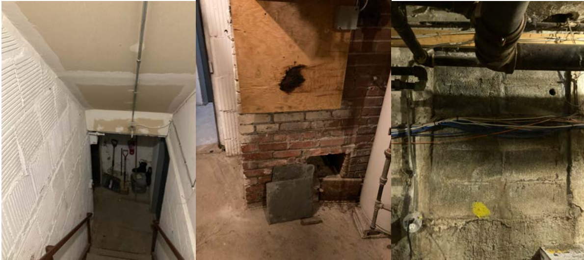
Stairwell to the basement and hollow clay tiles (L), brick chimney (C), concrete block foundation (R).
