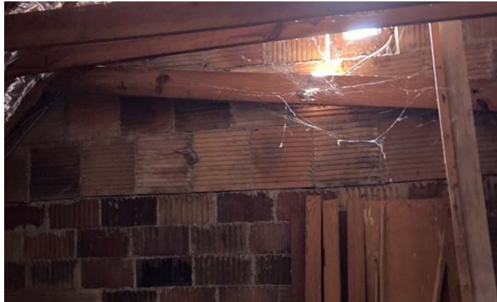
Downward movement in the center of the wall, and subpar mortar quality.
