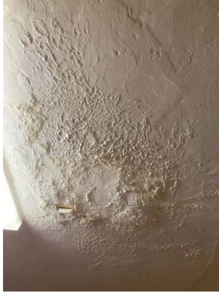
Severe plaster damage on the Jury Room ceiling.
