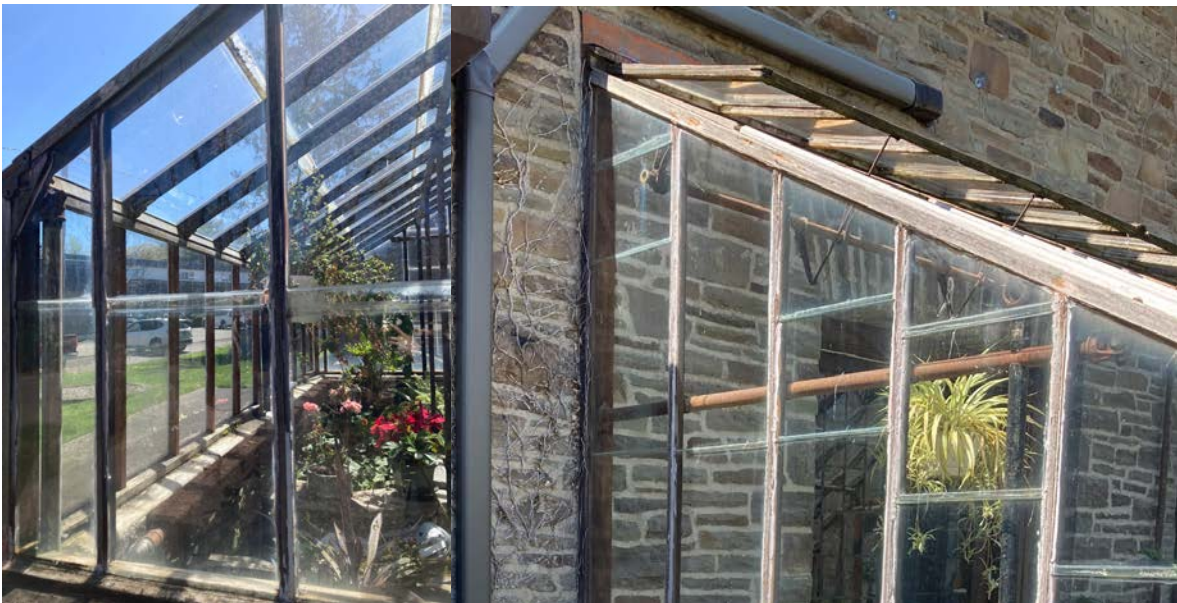
Deterioration of wood members (L) and rusting of the metal (R) around the greenhouse.
