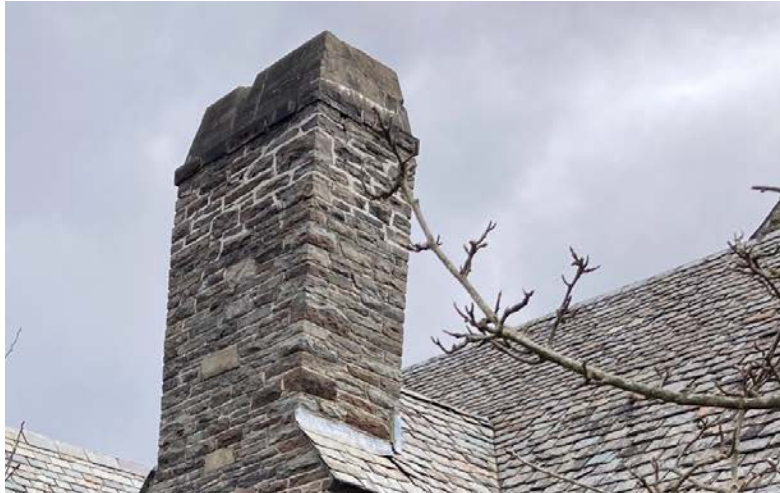
Deterioration of the upper part of the chimney between B and C.
