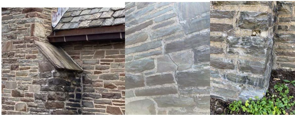
Moisture damage and staining (L), large cracks (C) missing mortar and stone and efflorescence striations (R), all on and around the chimney between Section B and C.
